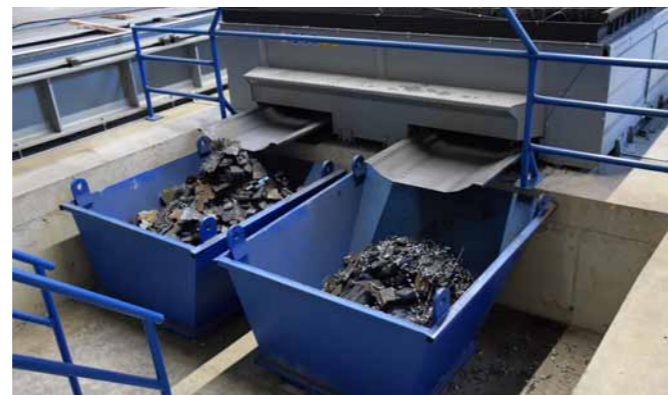
Today: ZINTRAC with automated slag disposal
